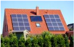
On-grid residential roof-tops
